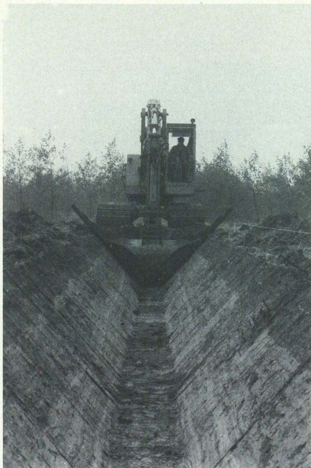
Fig. 7 Digging a ditch in the Holocene lagoonal Almere Member for scientific and educational purposes near the traffic circuit of the State Highways 50 and 338 in October 1979 in the Noordoostpolder (Overijssel).
