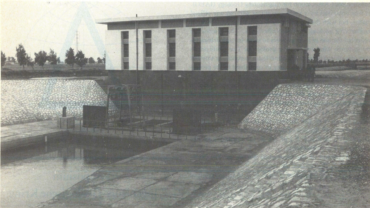
Plate I Pumping station Khandak el Gharbi in the delta of the Nile. This pumping station is one of the 64 pumping stations in the delta for removal of drainage water. Drainage is applied not for removal of excess water from rainfall, which is practically nil, but for salinity control. Through a subsurface drainage system consisting of tile drains the groundwater table is maintained at some 1.5 m below the surface and at the same time leaching of the soil with irrigation water is applied.
