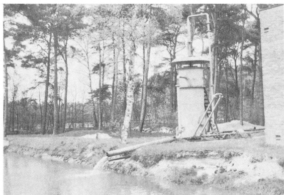
Fig. 24 Test filter for treatment of deep groundwater.
