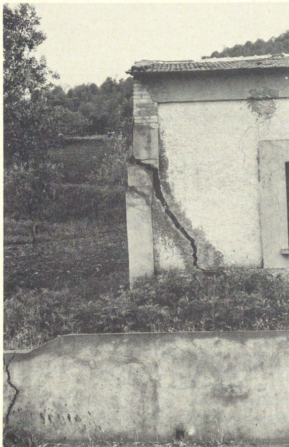
Fig. 1 House damaged as a result of sliding in marly clay.
