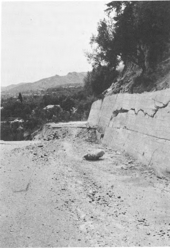
Fig. 8 Road destruction as a result of landslide opposite Rende (cf. fig. 7).
